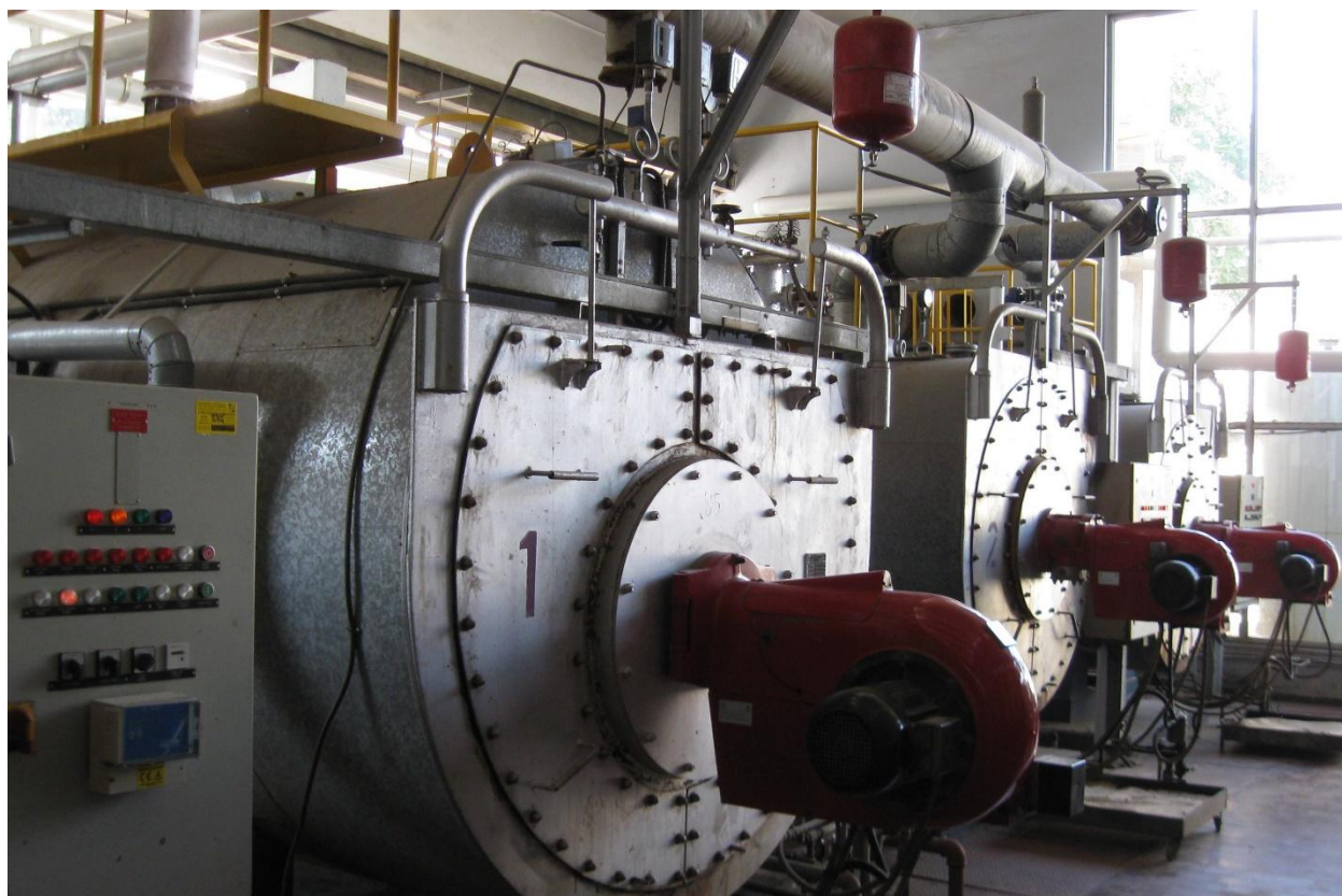
Fig. 7. Automatic line of industrial boilers with a capacity of 10 tons of steam per hour - each
