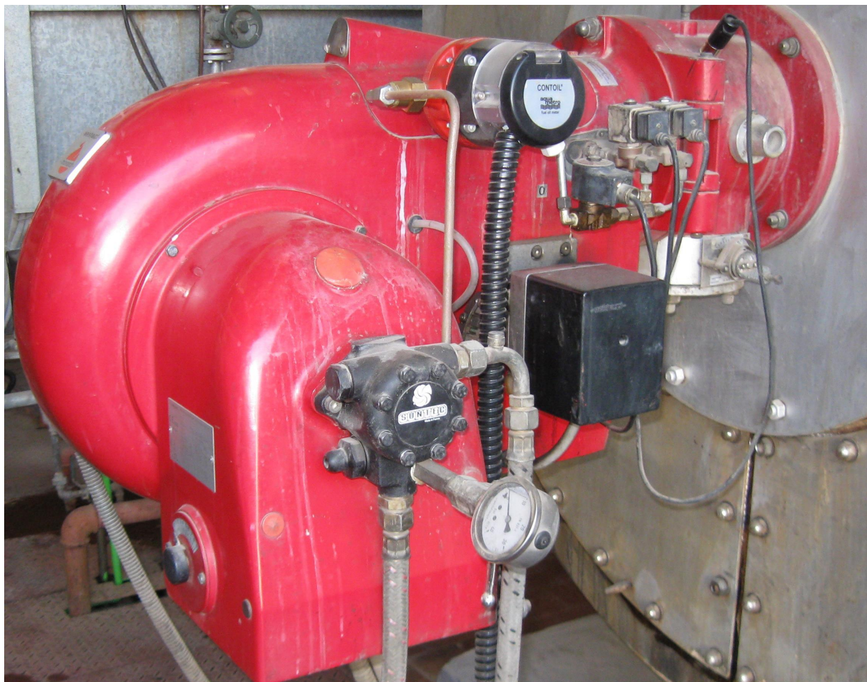
Fig. 6. Boiler control and monitoring system with a capacity of 10 tons of superheated steam per hour
